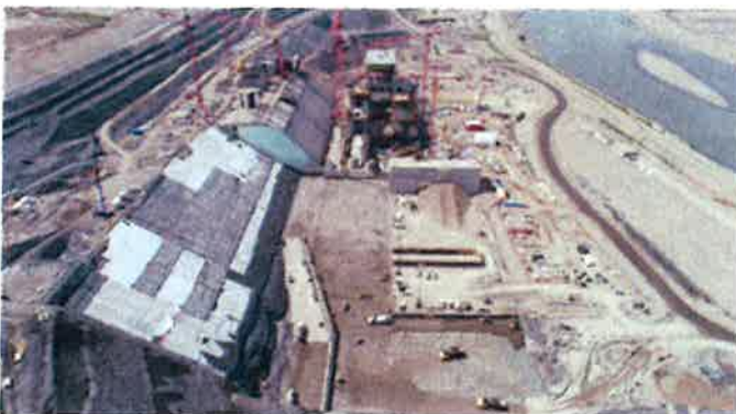
The Site C spillways excavation (foreground), powerhouse and main service bay, looking upstream, in July 2019.
