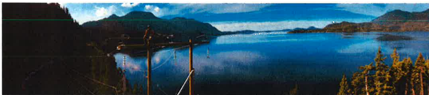
Dylan Martini, Power Line Technician, BC Hydro, working on the Kennedy Lake project takes a moment away from line work to pose for a photo on top of a new transmission structure near Kennedy Lake.
