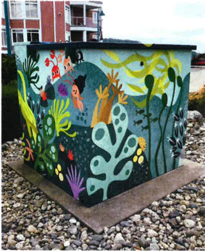
Decorative wraps on our pad-mounted equipment in Sechelt.
