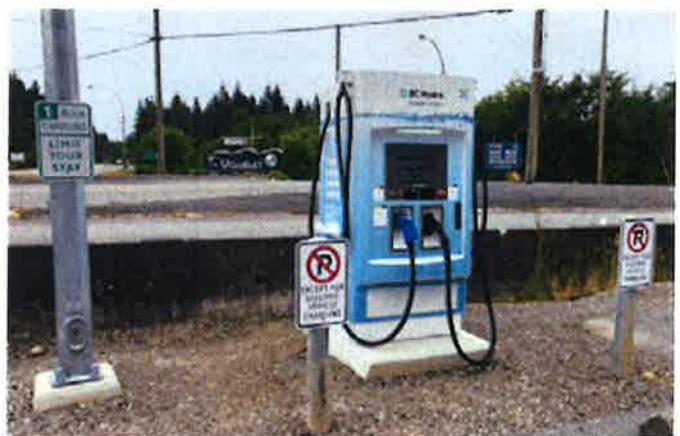
A fast-charging station installed at the Tofino-Ucluelet Junction.
