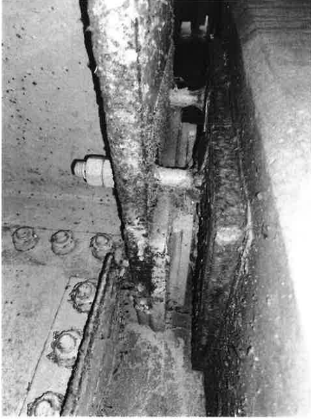
12 - Typical Bearing Corrosion
