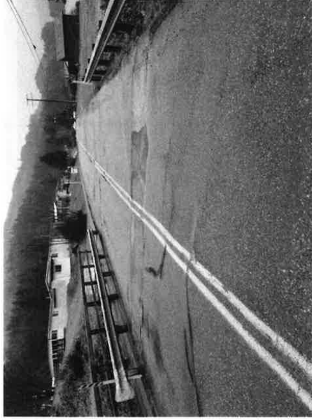
09 - Fill Settling North Abutment
