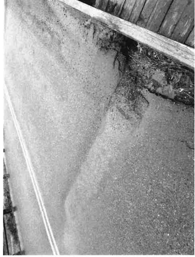
08 - Fill Settling Sound Abutment
