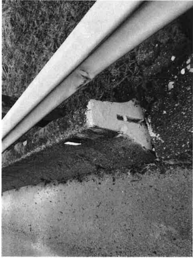
07 - Approach Barrier Connection
