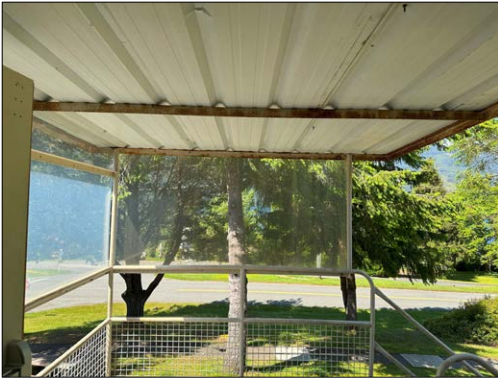
Photograph 1: Light rust to fire escape.
