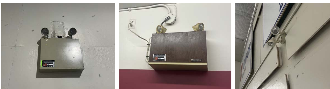
Figure 5: Examples of Emergency Lighting
