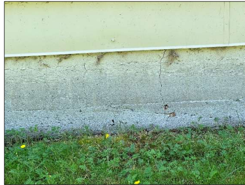
Photograph 8: Typical cracking to joints
