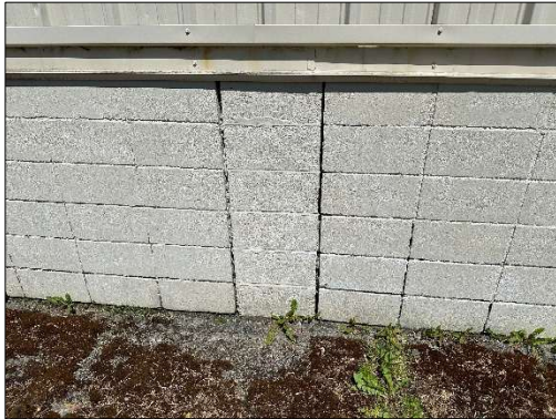
Photograph 7: Caulking missing at masonry foundation to north.
