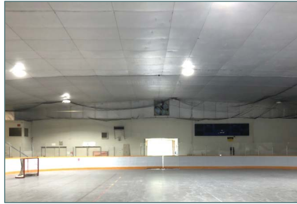
Figure 3: Roof insulation, bubble wrap type
