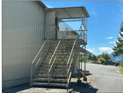
Photograph 2: Light rust to fire escape.
