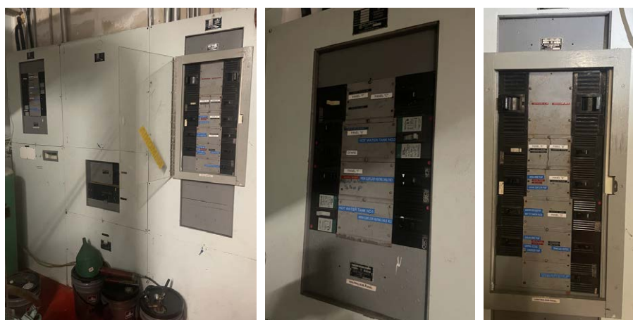
Figure 1: Canadian General Electric 1200 Amp Main Switchboard, 800 Amp Lighting Sub Panel & 400 Amp Heating Sub Panel
