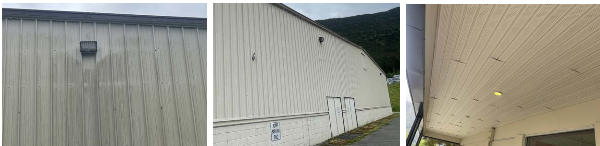
Figure 4: Examples of External Light Fixtures & Photocell
