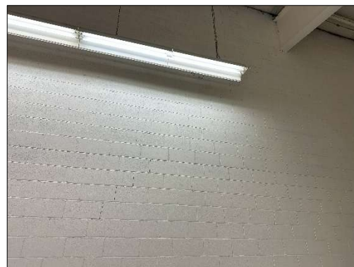
Photograph 12: Cracking to fire wall.
