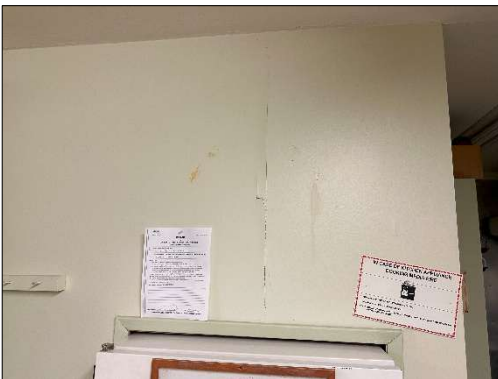
Photograph 3: Drywall cracking above fridge.
