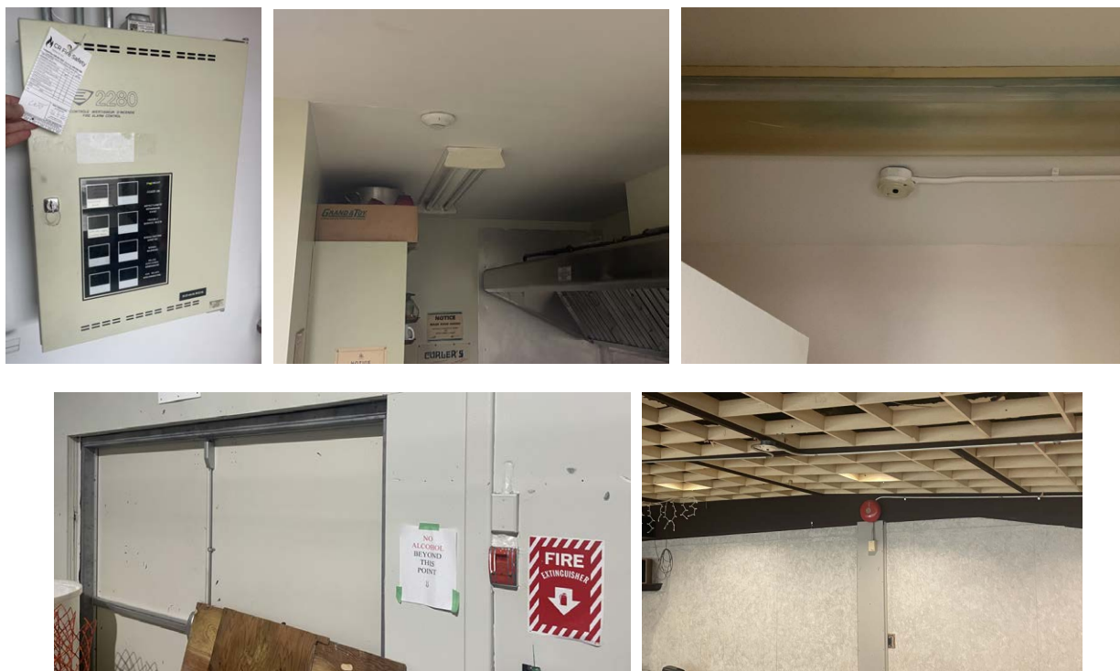
Figure 7: Fire Alarm Panel & Examples of Fire Alarm Devices
