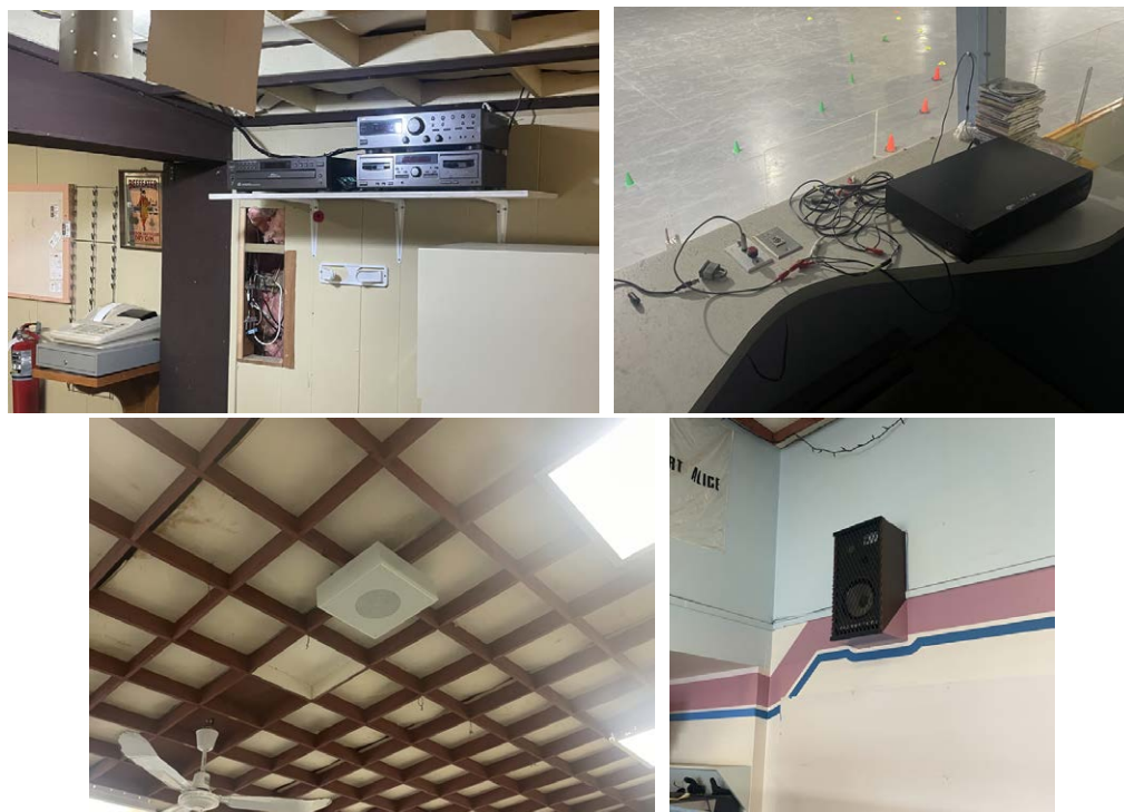
Figure 10: Examples of PA System Components
