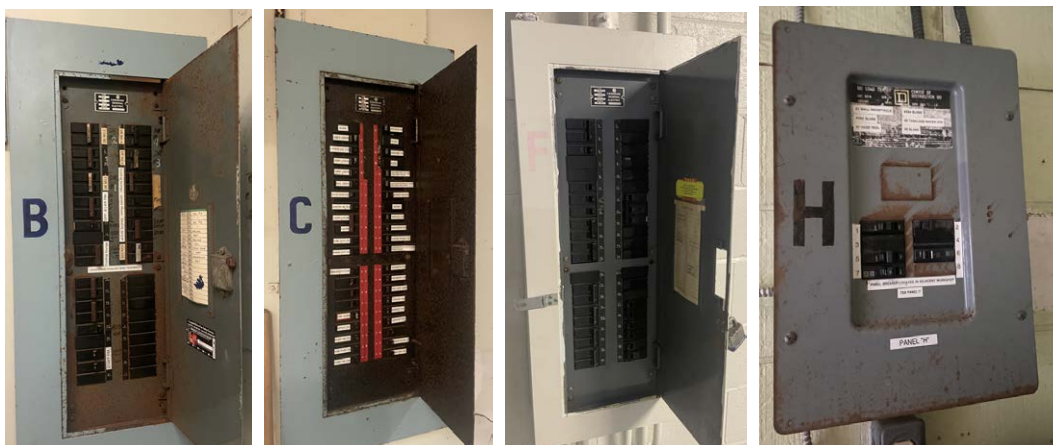
Figure 2: Examples of Distribution Panels; Evidence of Rusting
