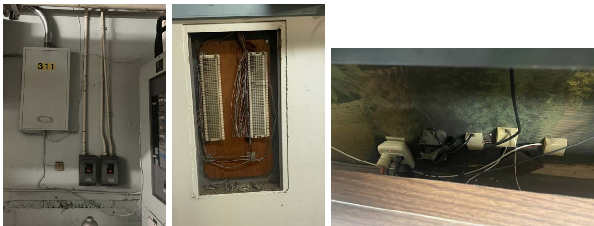
Figure 8: Telus Demarcation, Telephone / Data Tie In, & Telephone / Data Outlet Examples
