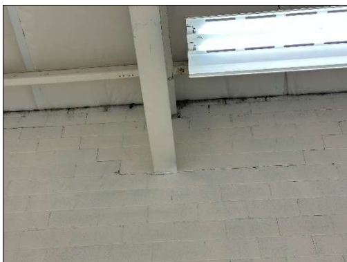
Photograph 11: Cracking to fire wall
