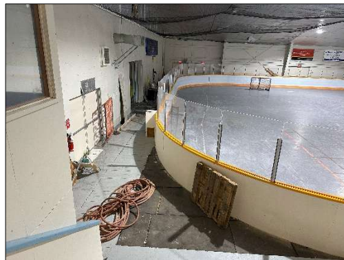
Photograph 4: Crack in ice slab indicating possible settlement.
